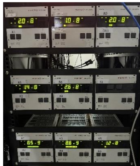
Fig. 7. Vacuum monitor panels
